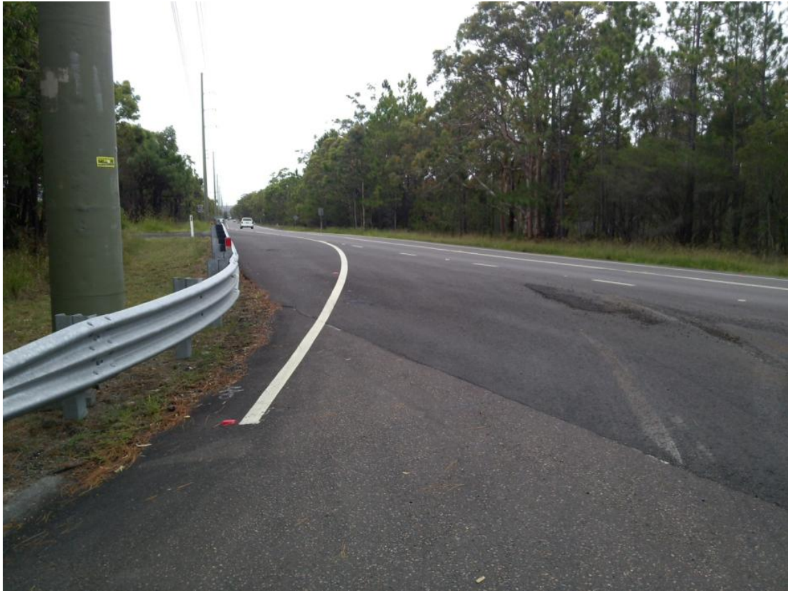
Photograph 7 – Ruttleys Road showing new guardrail and road shoulder south of the intersection
